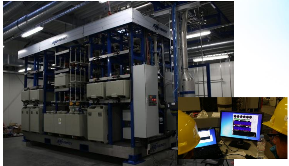
KORE producing electricity
