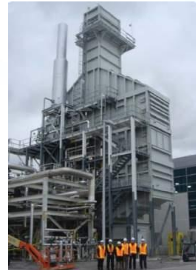
LMS6000 PD (derived from CF6-80C2), installed at Toronto airport for CHP (source: www.powerauthority.on.ca )
